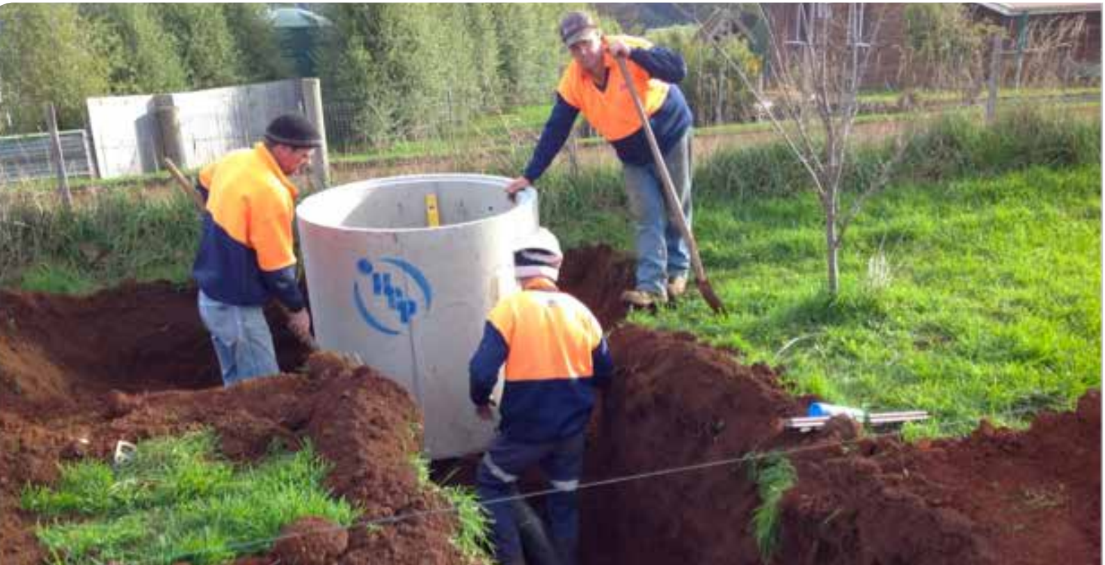
Figure 3: Air valve installation
