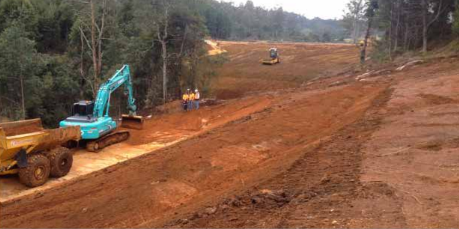
Figure 2: Excavation of the South Riana Dam pump station pad, downstream of the dam.
