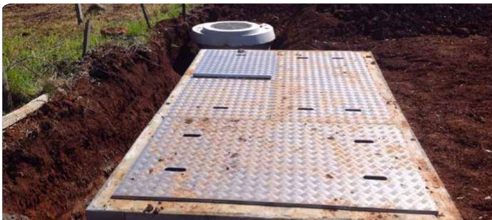
Figure 11: Pressure reduction valve pit West Pine
