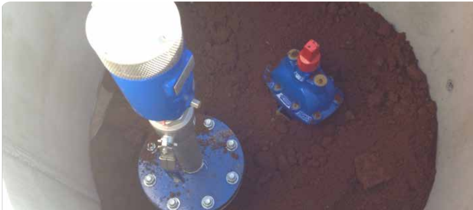
Figure 9: Isolation valve and air valve
