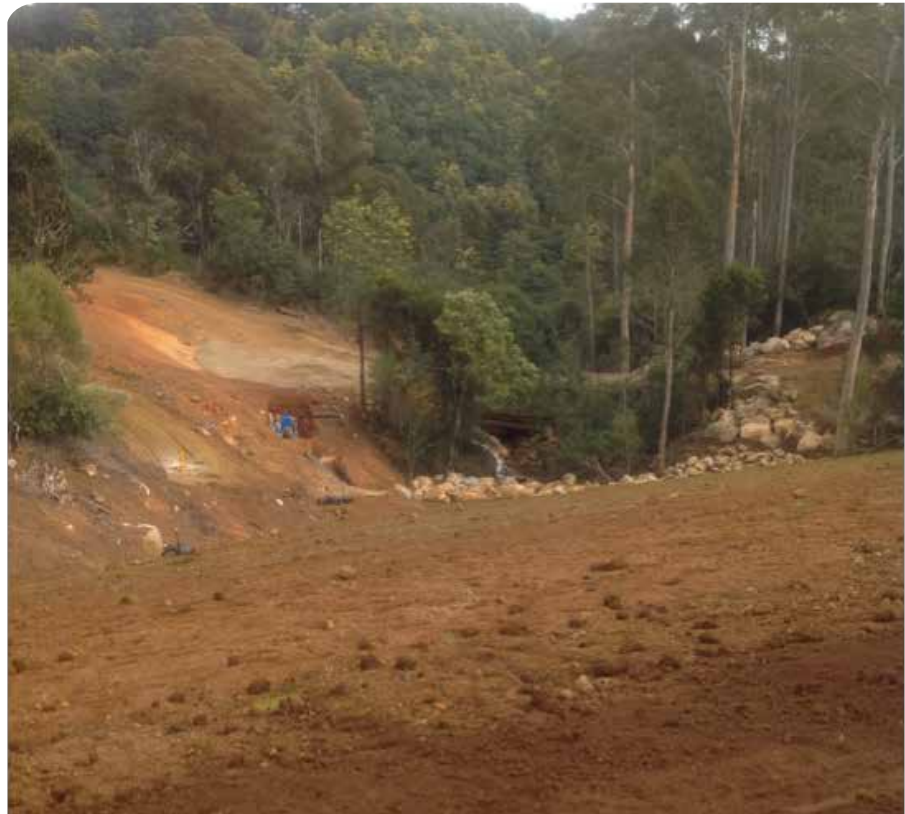
Figure 1: South Riana Dam pump station pad from the top of the dam wall
