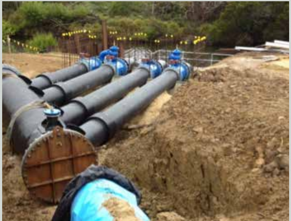
Figure 1: Pipe work at the Lower South Esk Pump Station
